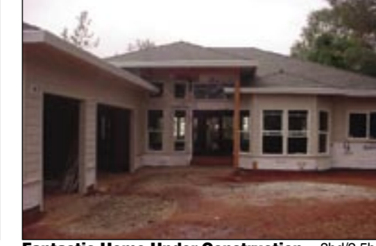
Fantastic Home Under Construction... 3bd/2.5ba in Penn Valley; popular floorplan w/great rm. + den; open kit. w/breakfast bar, granite counters, custom cabinetry and upgraded appliances. (MLS# 1022509) $739,500
